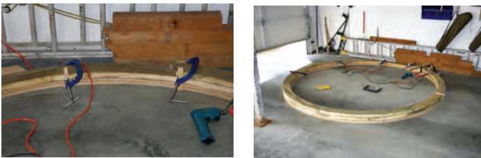
Figure 3 (left) — Fitting ring together Figure 4 (right) — Ring for base of observatory wall
