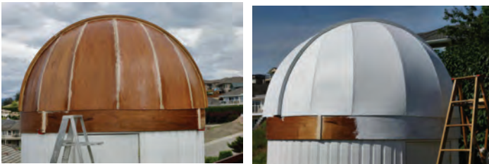
Figure 12 (left) — 1/4-inch mahogany plywood fastened and to be filled with Bondo and fiberglass Figure 13 (right) — Dome with several coats of ribs resin and paint.
