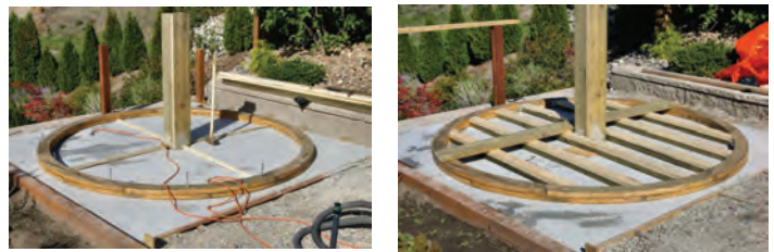
Figure 8 (left) — Base ring and pier installed Figure 9 (right) — Starting the installation of the floor.
